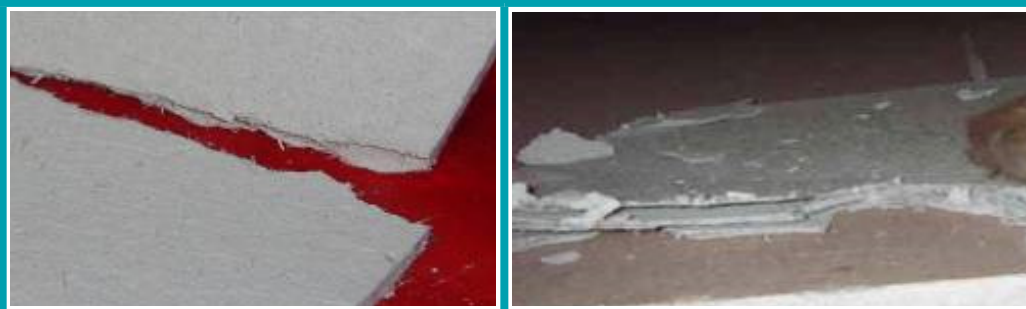
Figure 4 Ragged or torn edges of broken LDB
