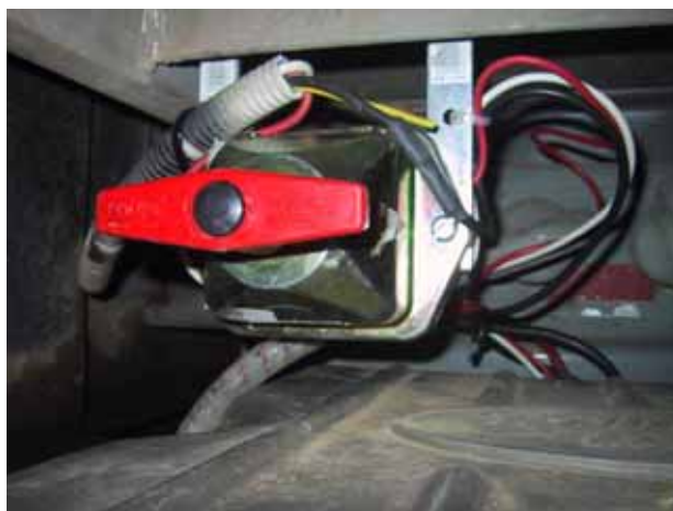
Figure 12 Installed Module Battery Isolation Switch (Shown in the OFF Position)
