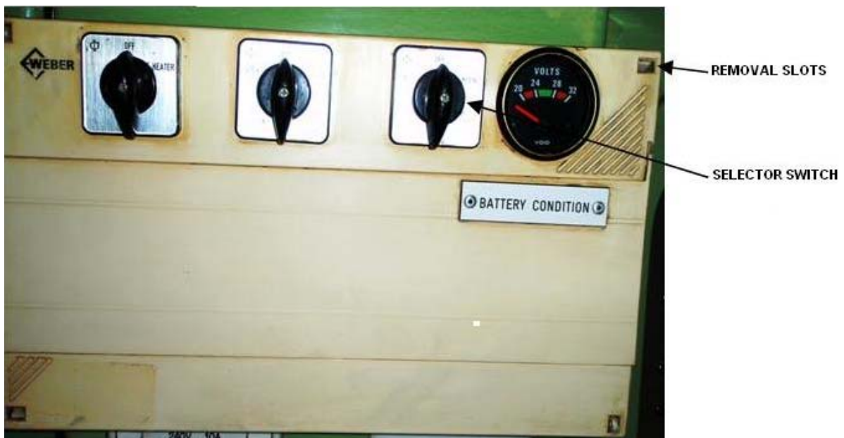
Figure 1 Switchboard Panel Cover
