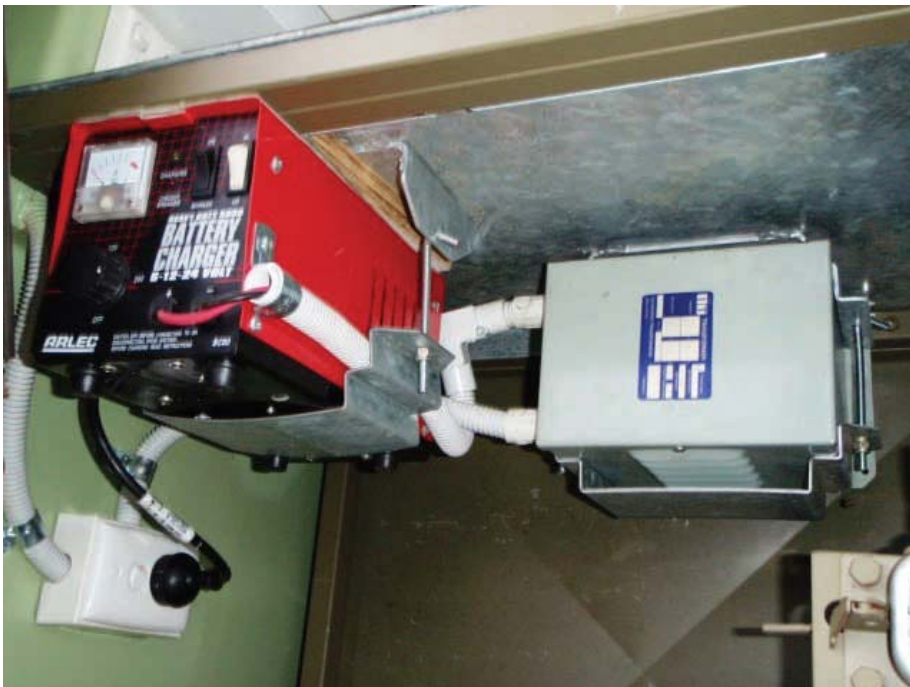
Figure 3 Original Battery Charger and Transformer
