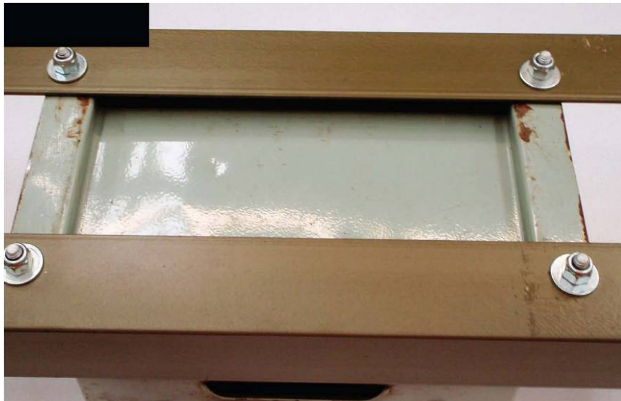
Figure 5 Transformer Mounting Nuts Secured
