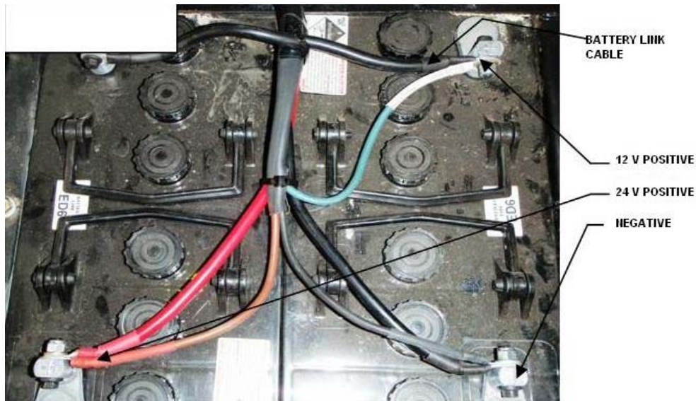
Figure 13 Wiring to Batteries
