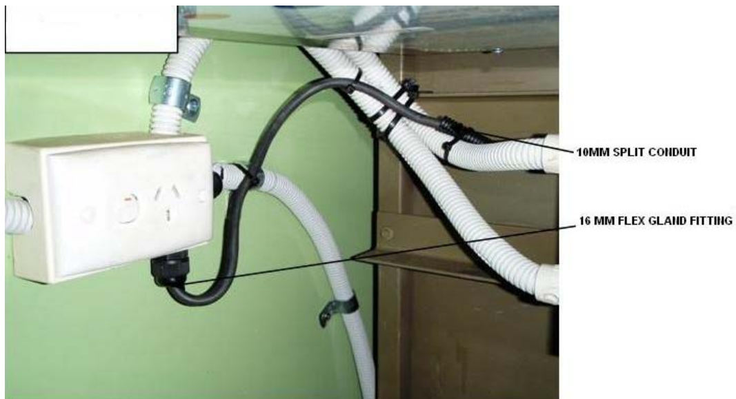
Figure 15 Battery Charger And Transformer Wiring Completed
