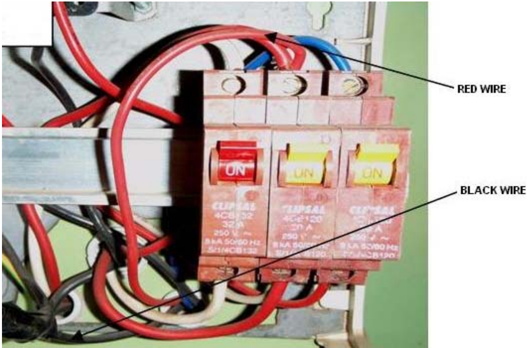
Figure 2 Battery Charger Wiring at Switchboard
