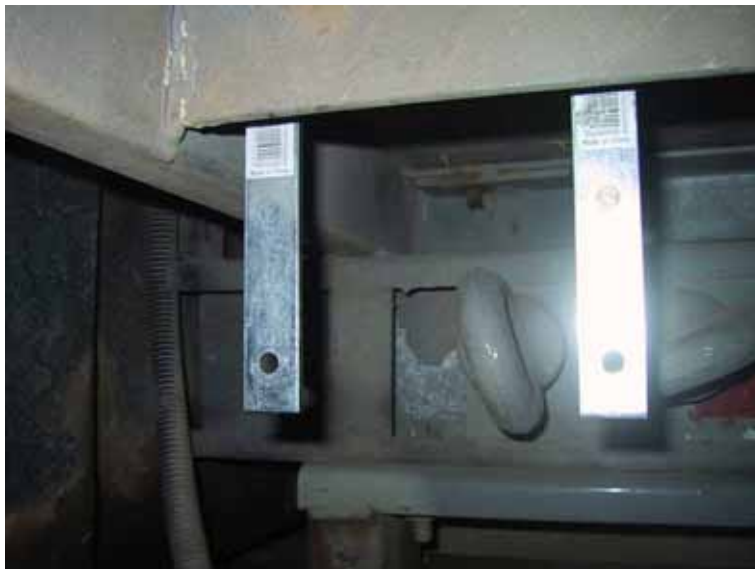
Figure 13 Isolation Switch Mounting Brackets Fitted
