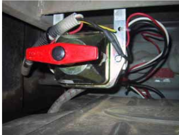
Figure 17 Installed Module Battery Isolation Switch (Shown in the OFF Position)
