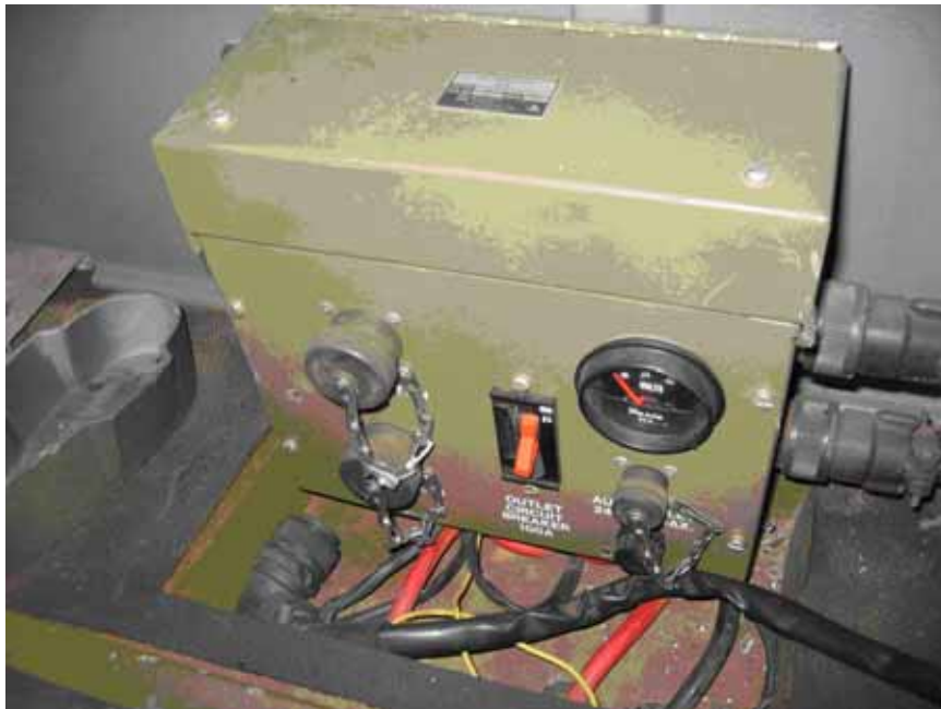
Figure 1 Power Distribution Panel Circuit Breaker
