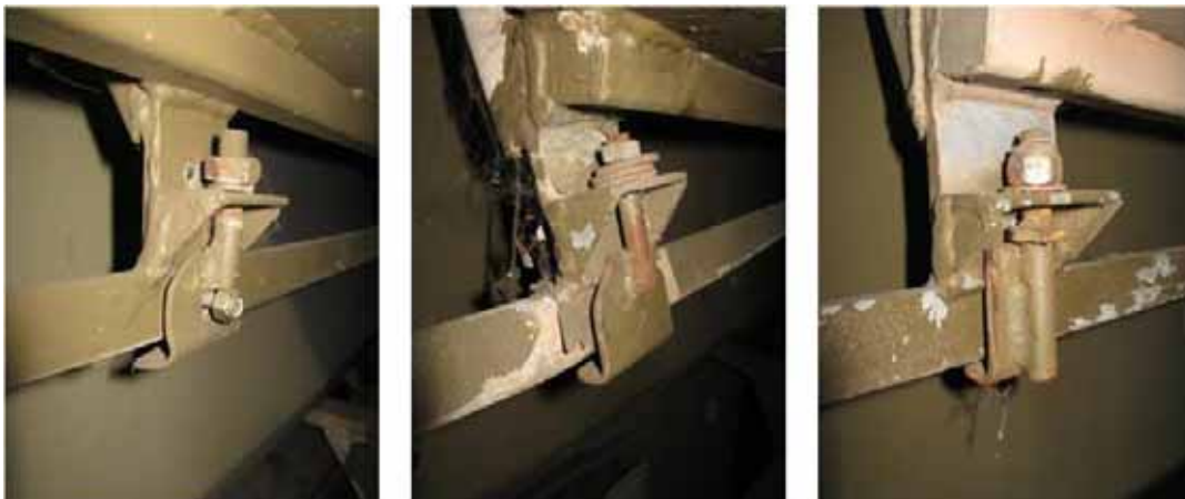
Figure 4 Incorrect and Modified Gutter Mount Clamps
