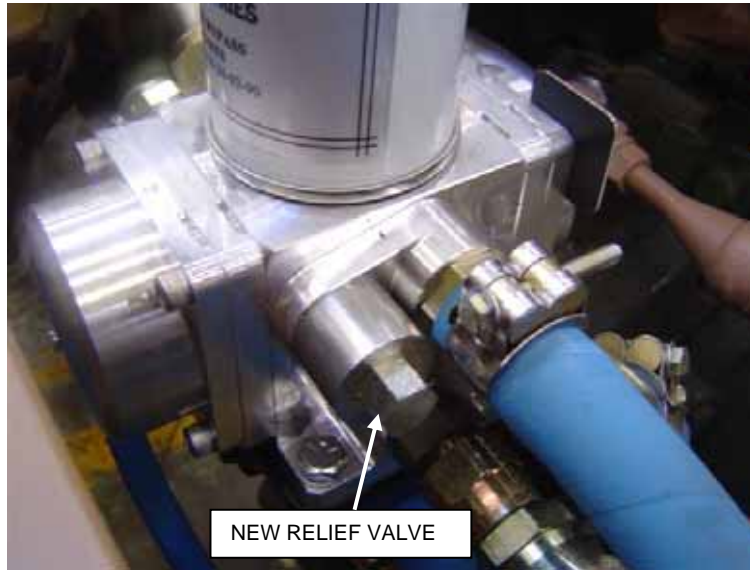
Figure 8 New Relief Valve Installed
