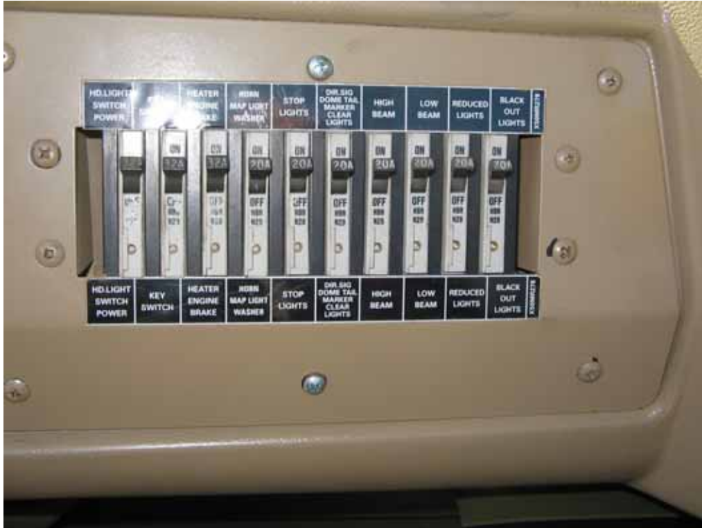
Figure 1 Existing Circuit Breaker Board
