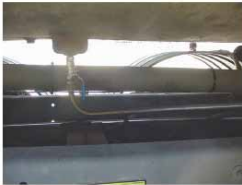
Figure 9 Centre Compartment Sampling Valve Tubes
