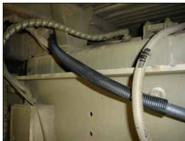
Figure 52 W2 Cable Adjacent to Left-hand Side Fuel Tank
