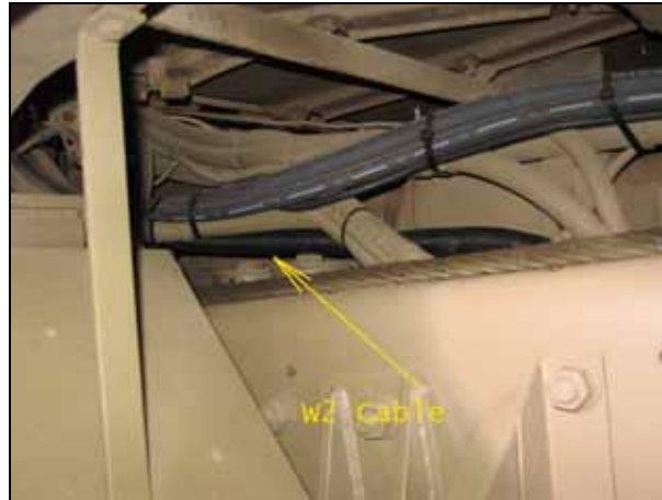
Figure 41 W2 Cable Route Under the Cabin, Left-hand Side
