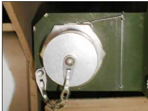
Figure 21 Cable Route to W1J1 Mounting Bracket
