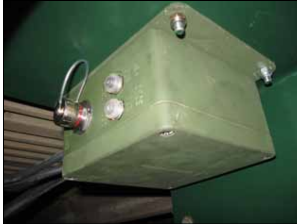
Figure 6 W1 Circuit Breaker Box
