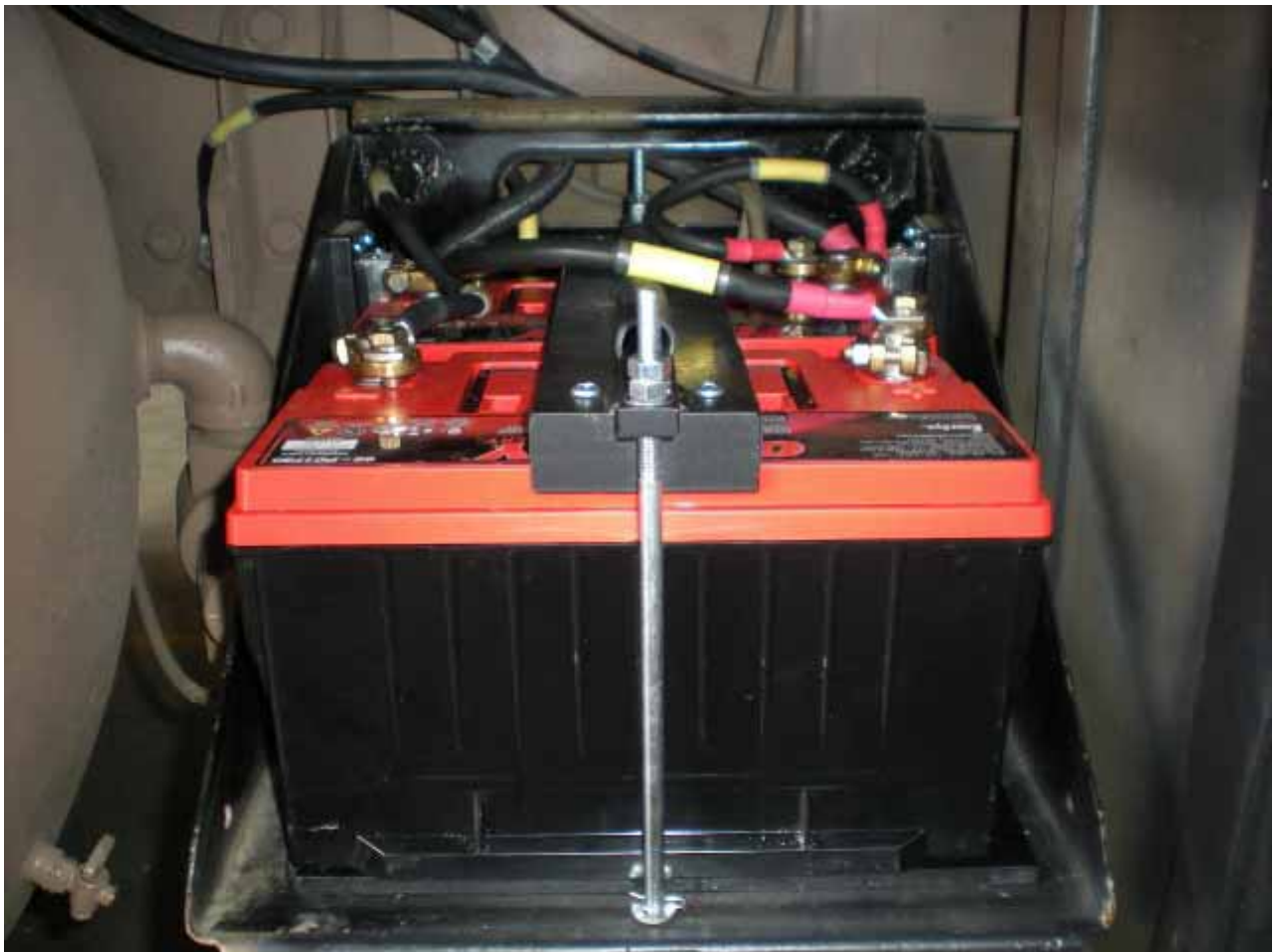
Figure 9 Battery Orientation and Connections - 2
