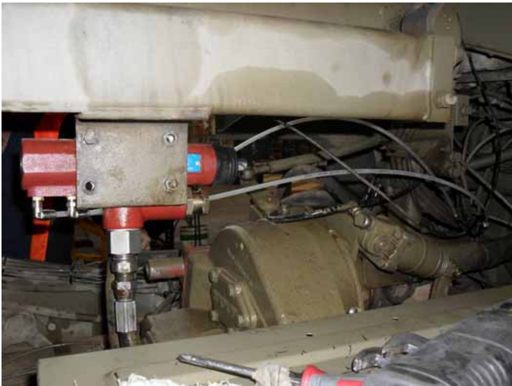
Figure 4 Air Lines Connected to Replacement Control Valve
