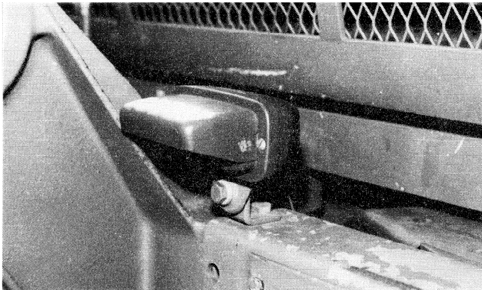
Figure 2 - Additional Blackout Light (Fitted Location)
