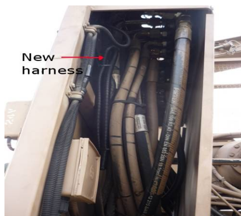
Figure 24 Harness under Control Panel
