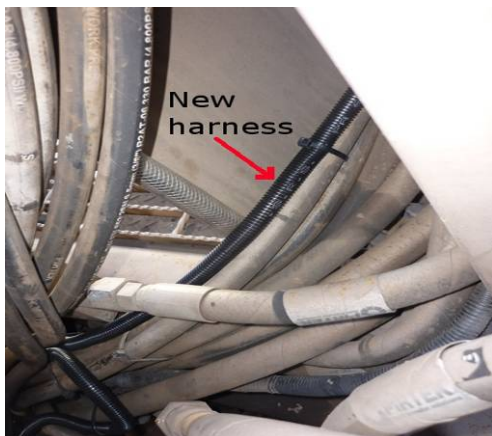
Figure 23 Harness at Control Platform
