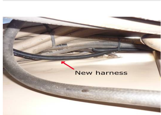
Figure 14 Harness at Operator Platform
